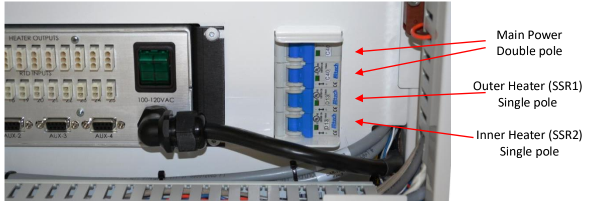
Main power circuit breaker for the S300 (e-box cover removed)
